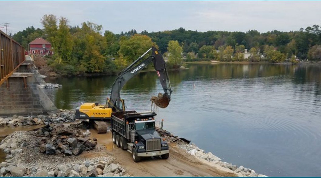
A causeway is built to facilitate construction access at the last minute due to the river draw-down.
