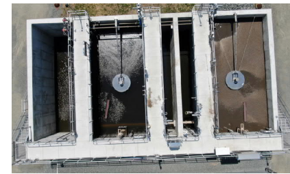
Sequencing Batch Reactors (SBRs)
