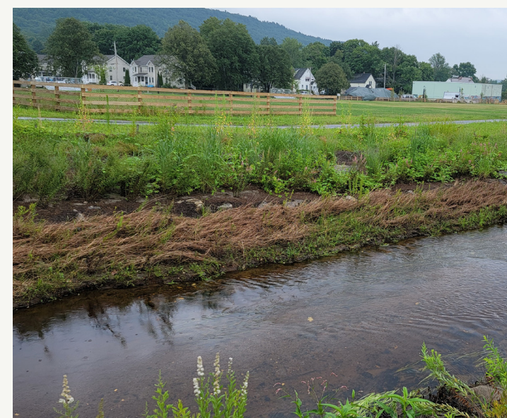
New revetment bank stabilization was incorporated along a portion of Beaver Brook.
